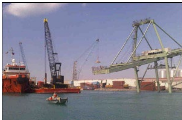
Main cargo moving crane in Port au Prince. The crane and the pier were destroyed during the January 12th earthquake. Resolve Marine is working to have this crane removed before beginning to work on the piers.
